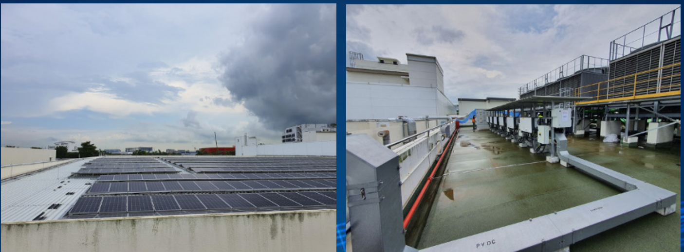
Figure 7.0 Example of a Large-Scale Solar PV Installation
